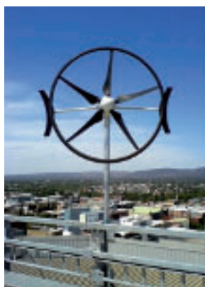
Figure 32 • 1.5kW mini-wind turbine above Wakefield House
