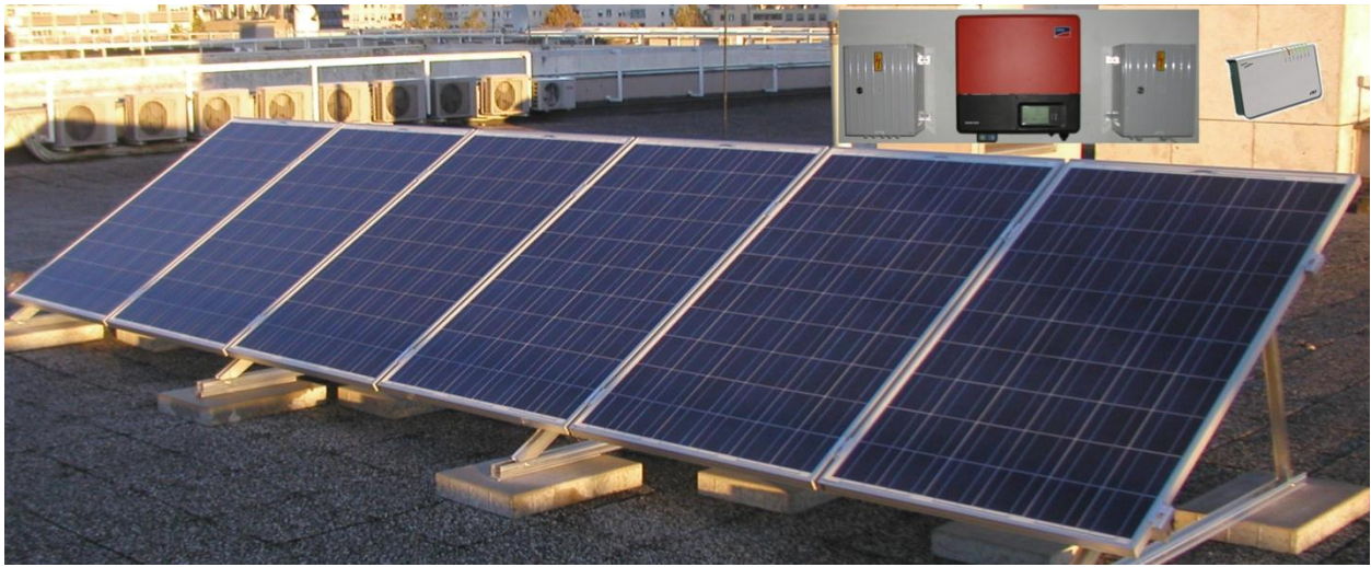
Figure 22 Photovoltaic system PV1kW_D connected to the grid (RE1)
