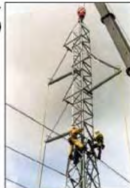
66 kV => 220 kV (Union Fenosa - Spain)
