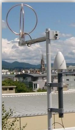
Lightning sensor measures magnetic flux in time in frequency range (1 kHz – 200 kHz)
